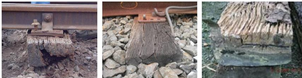
(a) Fungal decay
