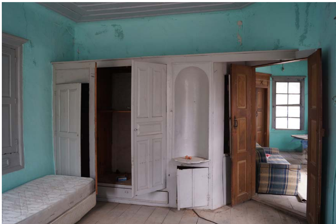
Fig. 5. A cupboard and a lamp niche in the wall opposite the hearth.
